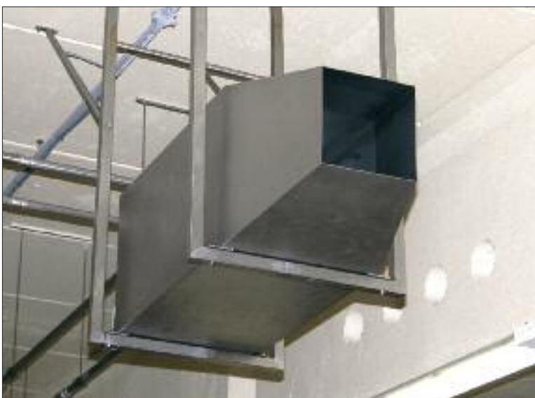
One of the circulation fans used to optimize the air flow.
