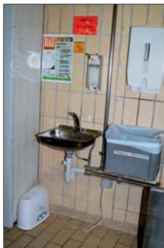
An additional small air degermination unit (below left) has been placed in this sensitive personnel hygiene area
