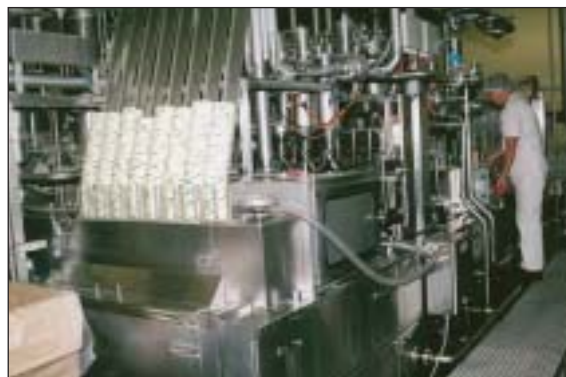
With air degermination measures almost aseptic conditions can be achieved at this 13-year-old filling and closing unit for yogurt products.
