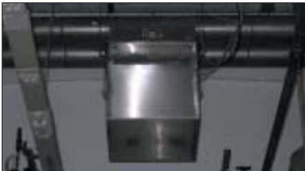
Fogging unit underneath the ceiling at Schlütter.
